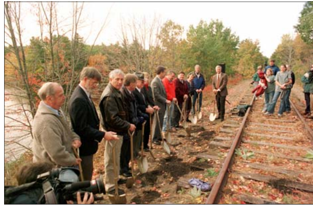
Following eight years of planning for the Mountain Division Trail, local and state officials break ground on October 22, 2002.
